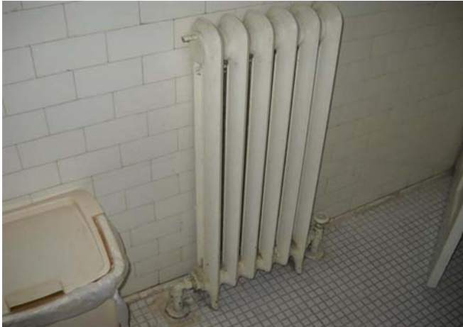
Photograph No. 19 Typical radiator located in Baxter House.
