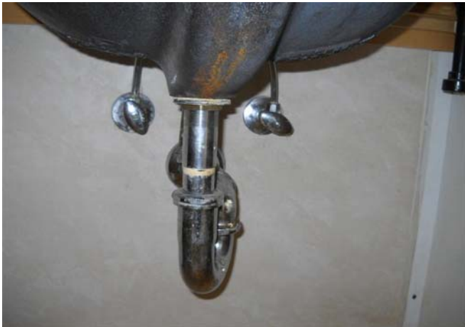
Photograph No. 39 Typical piping under sinks at the main church building.
