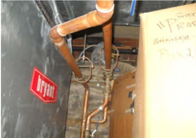
Photograph No. 37 Typical copper piping at the main church building.
