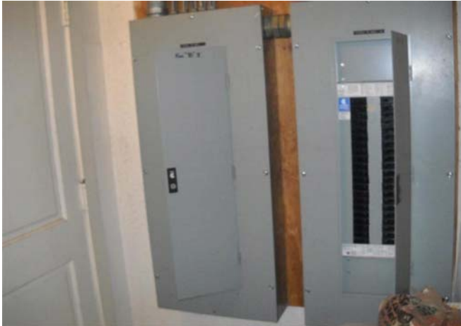
Photograph No. 25 Typical electrical panel located in the undercroft.
