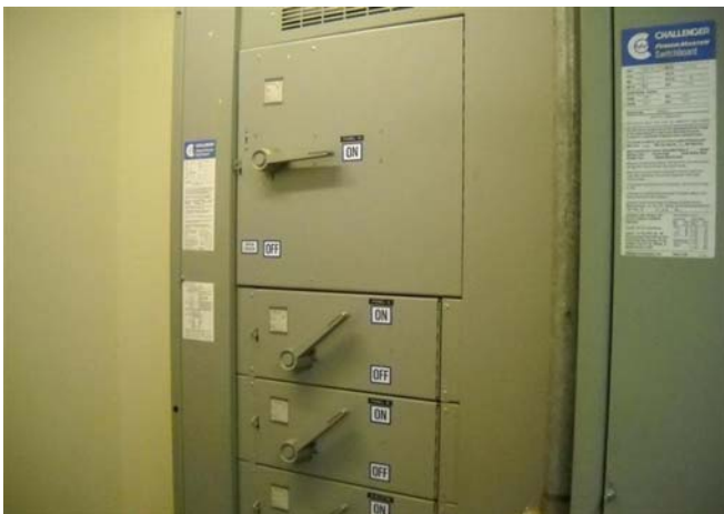
Photograph No. 23 Main electrical cut-off switches in the main church building.
