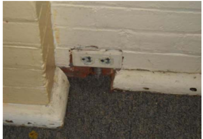
Photograph No. 28 Damaged electrical outlet in the conference room in the main church building.
