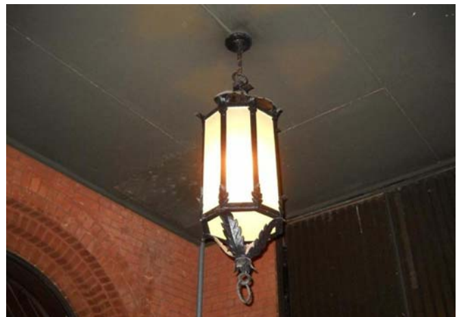
Photograph No. 30 Typical light fixture in the nave.
