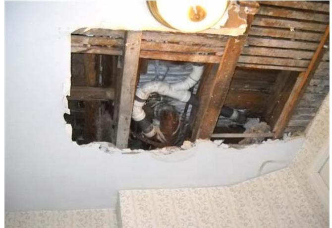
Photograph No. 46 Leaking waste piping exposed by a damaged ceiling on the first floor at Baxter House.
