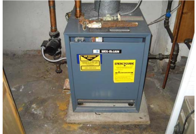
Photograph No. 20 Boiler located in the basement of Baxter House.
