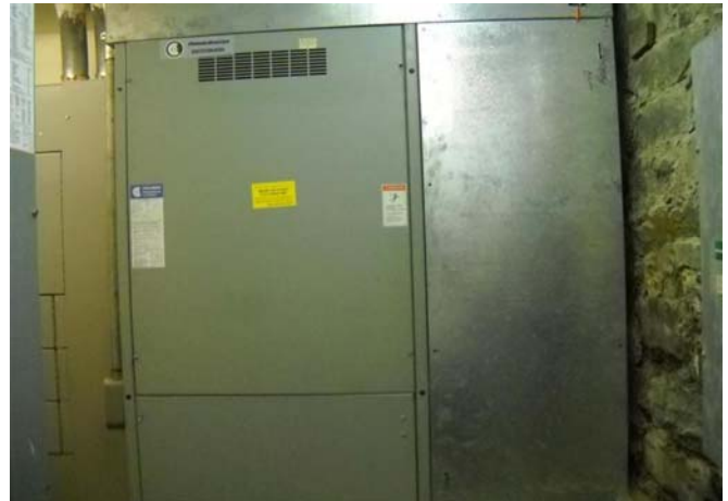
Photograph No. 22 Main electrical panel at the main church building.
