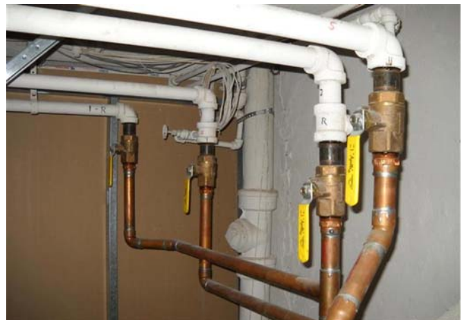
Photograph No. 48 Typical pipe work in the basement of Baxter House.
