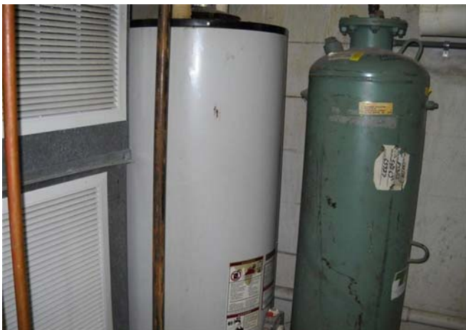
Photograph No. 41 Water heater in the main mechanical room in the undercroft of the main church building.
