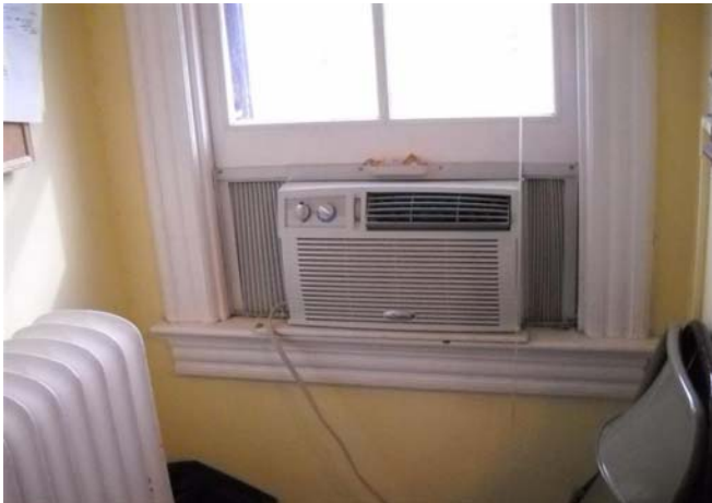
Photograph No. 21 Through-the-wall air-conditioning unit in a second floor office at Baxter House.
