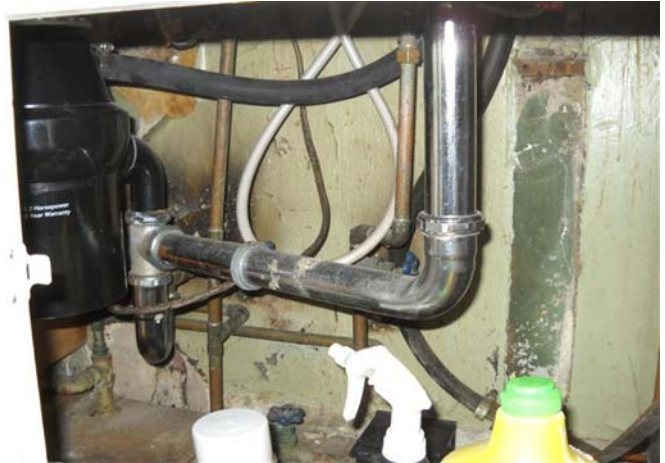
Photograph No. 44 Typical waste and supply piping at Baxter House.
