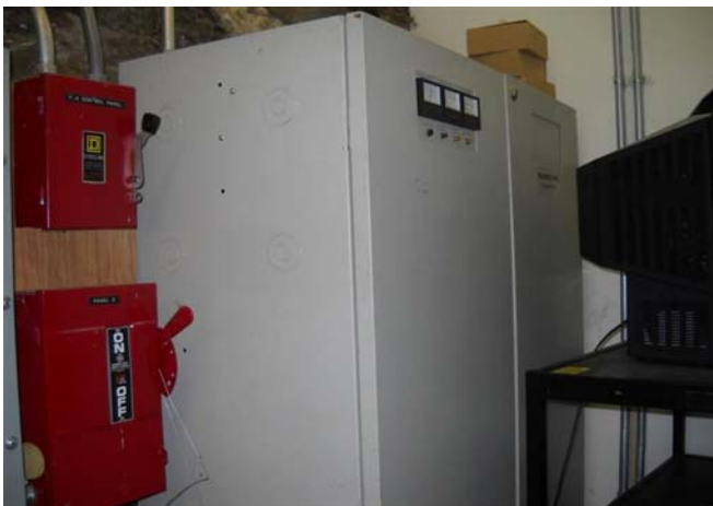
Photograph No. 29 Emergency power panel in the electrical room in the undercroft of the main church building.
