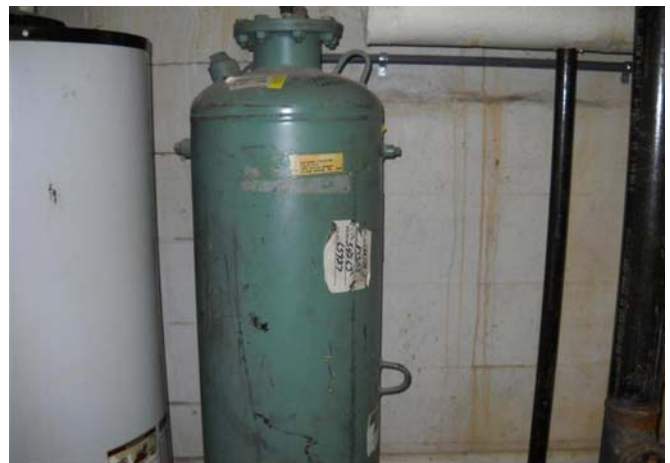
Photograph No. 42 Compression tank for the water heater in the main mechanical room.
