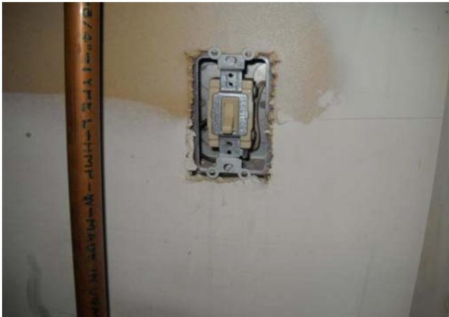
Photograph No. 27 Open electrical switch in the undercroft at the main church building.
