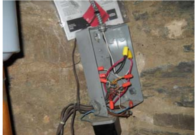
Photograph No. 26 Open electrical box in the mechanical room in the parish hall.
