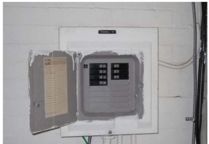
Photograph No. 24 Typical electrical panel located in the parish hall.
