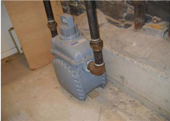
Photograph No. 43 Main gas entrance and meter at the main church building.
