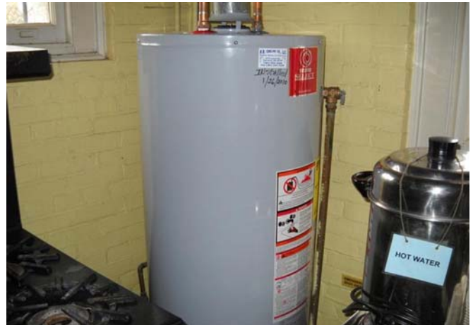
Photograph No. 40 Water heater in the kitchen at the parish hall.
