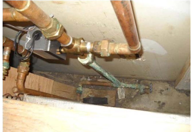
Photograph No. 38 Leaking and damaged copper piping in the undercroft of the main church building.
